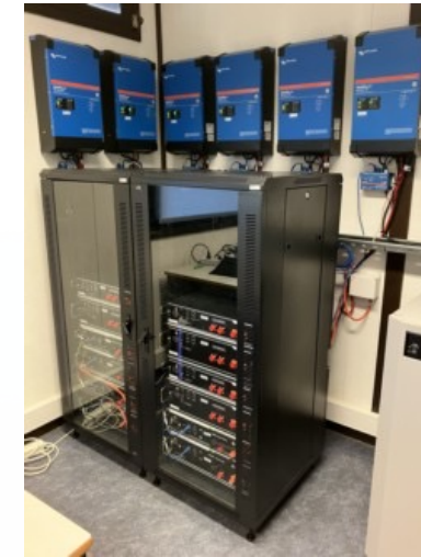
Energy Storage System with six batteries
